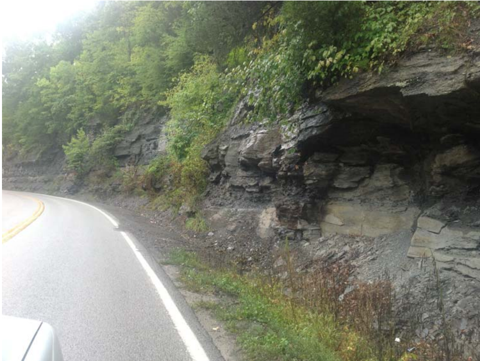
Existing cut slope in Breathitt Formation showing undercut due to highly weatherable shales
